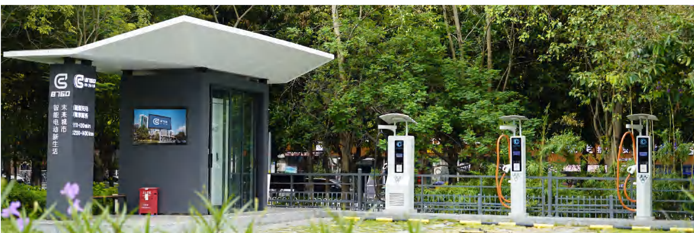
Industrial Park Super PV-Energy Storage-Charging Pile Station
