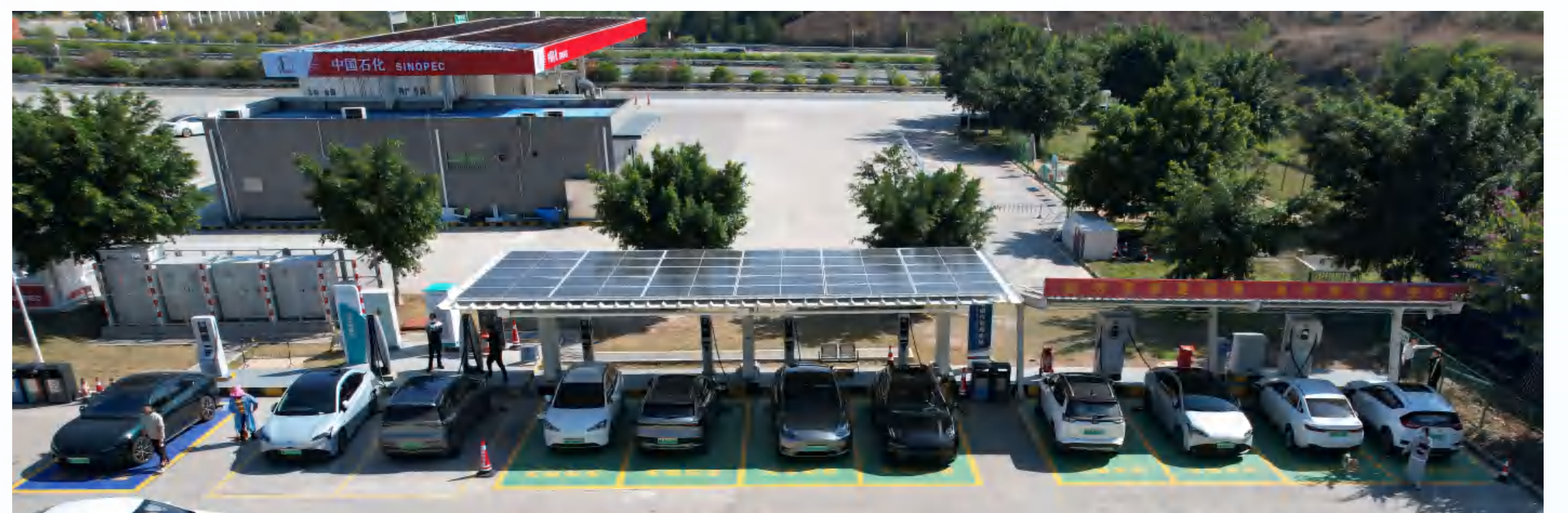
PV-Energy Storage-Super Charging Station In Highway Service Area
