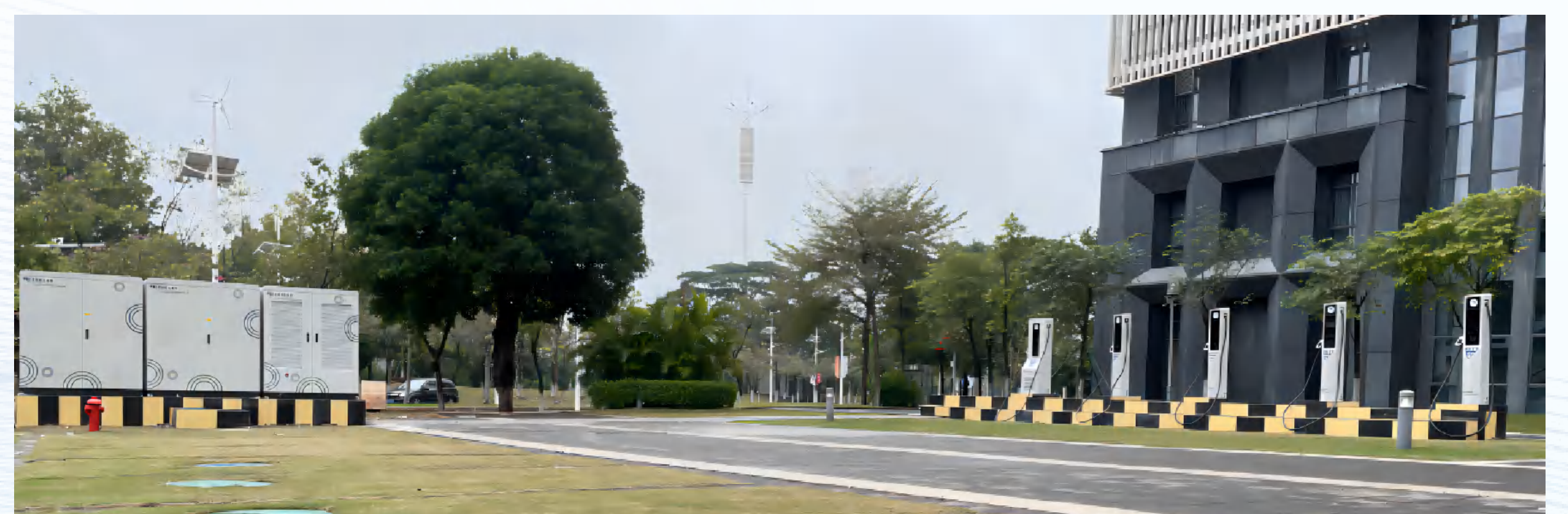
Guangzhou Bio Island Energy Storage and Super Charging Station
